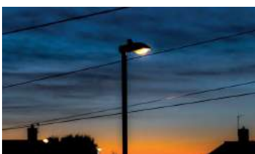
3. Street light sensor
